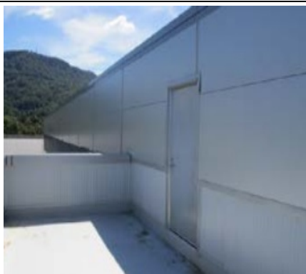
South East Terrace Access Door access via the plant room
