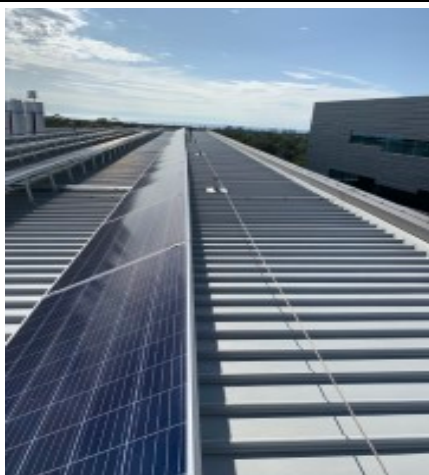
Upper Roof area with solar panels and lifeline (Certification by Riverlands Roofing Status Current)
