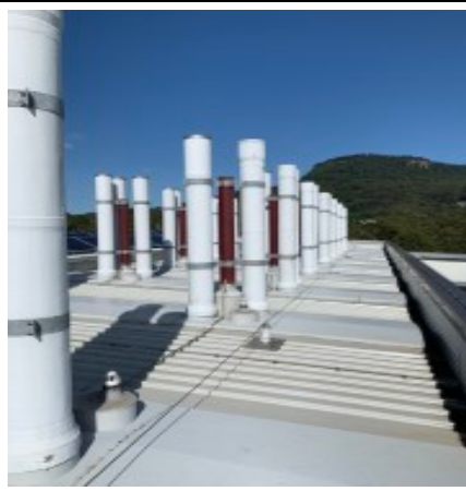
Upper Roof lifeline and fume cupboard exhaust stacks (Certification by Riverlands Roofing Status Current)
