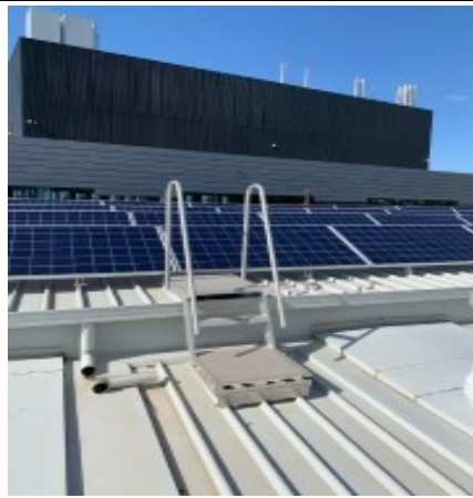
Upper Roof area with solar panels and fixed ladder
