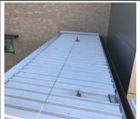
Bridge Link to Building 41 only accessible by EWP Lifeline & Anchor points Currently not Certified & must not be used
