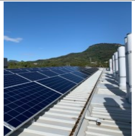
Upper Roof area with solar panels
