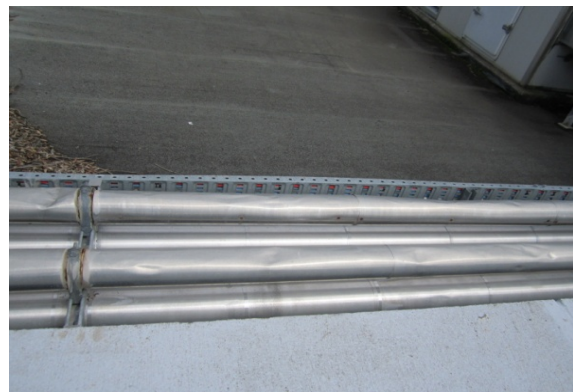
Pipework on roof
