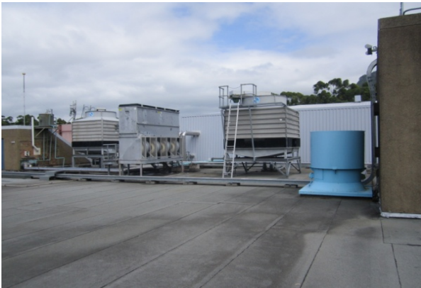
Cooling towers in centre of building and secondary access stairs
