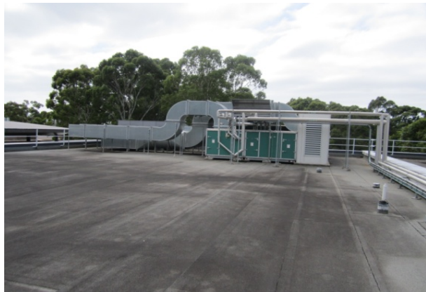
Airconditioning unit on northern side of building
