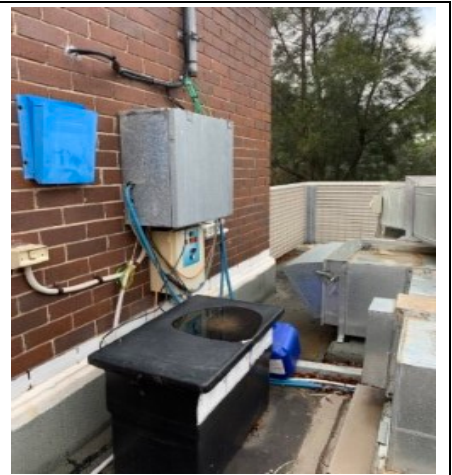
Building 2 roof area with cooling tower chemical storage
