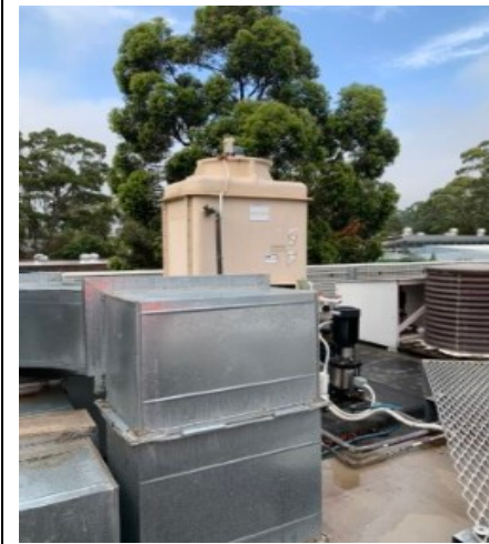
Building 2 roof area with ducts and cooling tower and walkway
